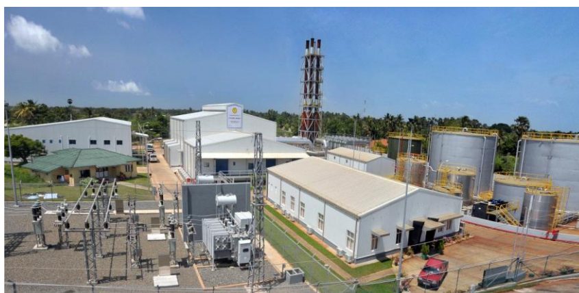
Fig 8 – Uthuru Janani 24 MW Thermal Power Plant Line
