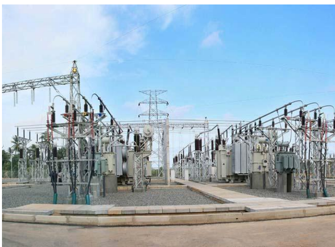
Fig 4 – Chunnakum Grid Substation
