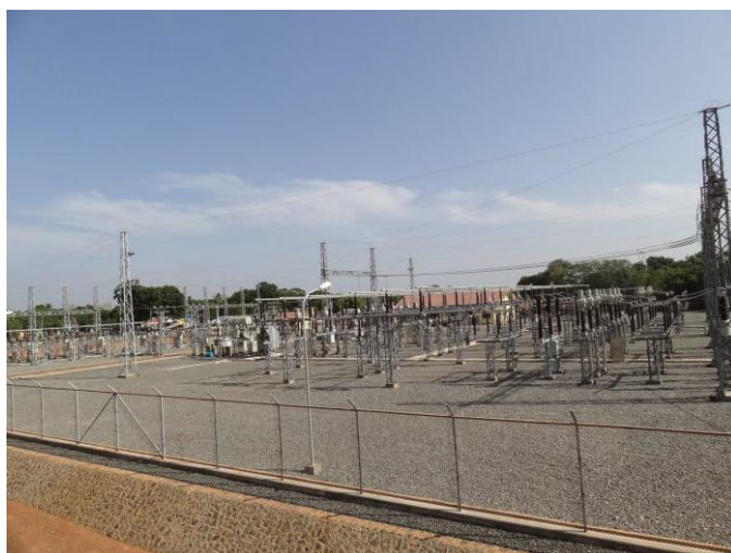
Fig 5 – Kilinochchi Grid Substation
