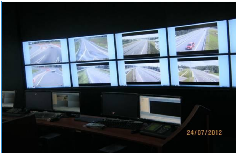
Video Monitoring system
