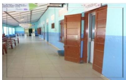
Modernization of Jaffna Hospital
