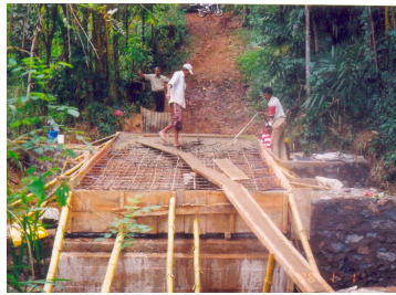
Ongoing Development of the Lorawatta Bridge belongs to the Panwilathenna Grama Niladari Division in the Doluwa Division of the Kandy
