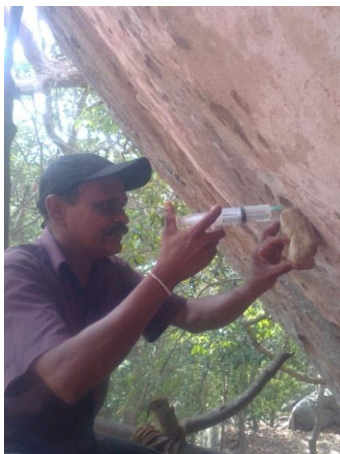
Chemicals are being injected to the mortar in order to reinforce it.
