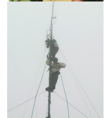
Maintaining radio communication system
