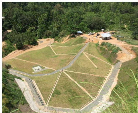
Site view from Upper area at A005-167 at Lunugala,(Construction of surface drainage, Surface drainage, drainage well and underground horizontal boring)
