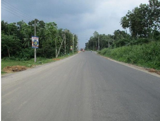
Miscellaneous Foreign Aided Project, Improving Kotte – Bope Road (Wearing course laying at Ch 4+900)
