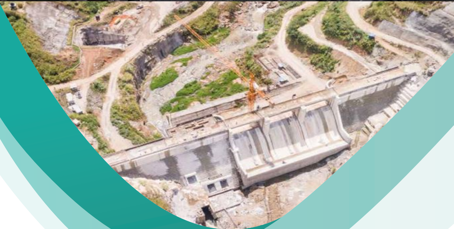
POWERHOUSE & TRANSFORMER CAVERN Type of Turbines: Pelton 2 Unit: 60 mW Capacity: 120 mW
