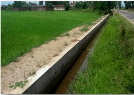
Improvements to Structures in Muslim Kolaniya DCO in D2 Main Canal Part 01 (RB - 06) - Polonnaruwa
