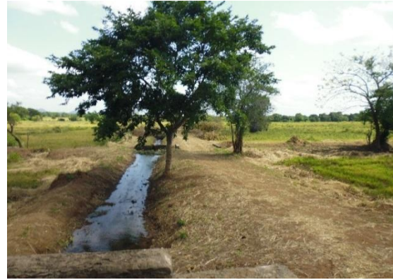
Distributory Canal maintained by sharamadana under Social Security Program of Dam Safety Project - Maha Kanadarawa Scheme
