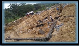
Construction of two storied building for Sri Pada Pilgrim's Rest in Sri Palabaddala
