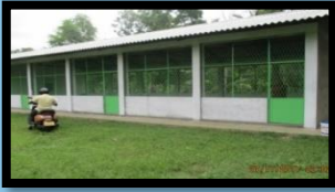
Colour wash and power supply for the Community hall at Medabedda Colony in Balangoda (DCB)
