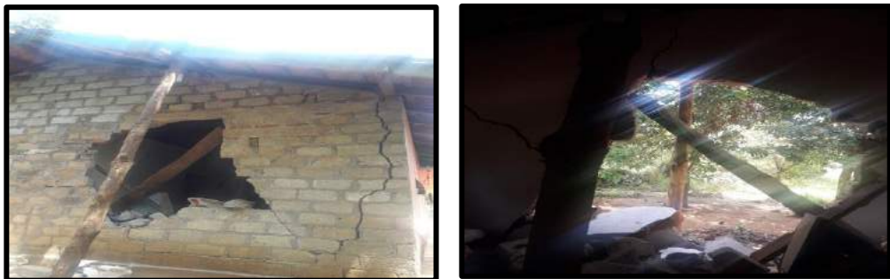
Damages caused to Houses by Wild Elephants in DS Division, Minipe
