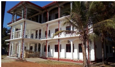
Construction of New office building at the cost of 57.8m for DS office, Koralaipattu
