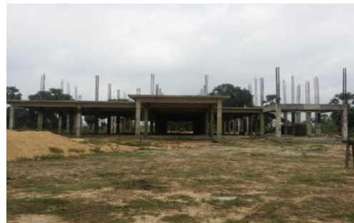
Construction of New office building at the cost of 80m for DS office, Koralaipattu West
