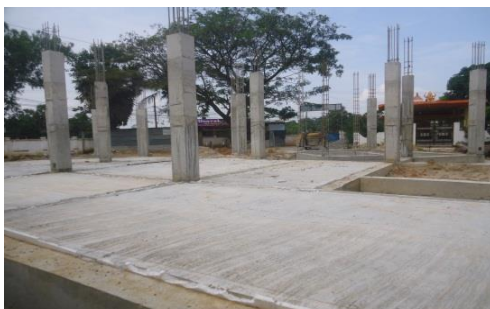
Construction of New office building at the cost of 120.76m for DS office, Manmunai .South Eru.pattu
