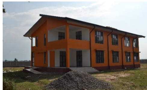
Construction of New office building at the cost of 49.3m for DS office, Manmunai south west
