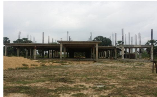
Contr. of New office building at the cost of 80m for DS office, Koralaipattu West
