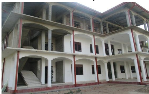
Contr. of New office building at the cost of 57.8m for DS office. Koralaipattu
