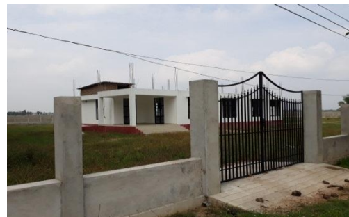
Contr. of New office building at the cost of 49.3m for DS office, manmunaisouth west
