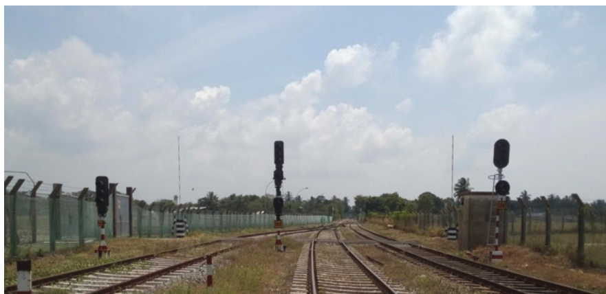
Signalling system installed at Katunayake Railway station
