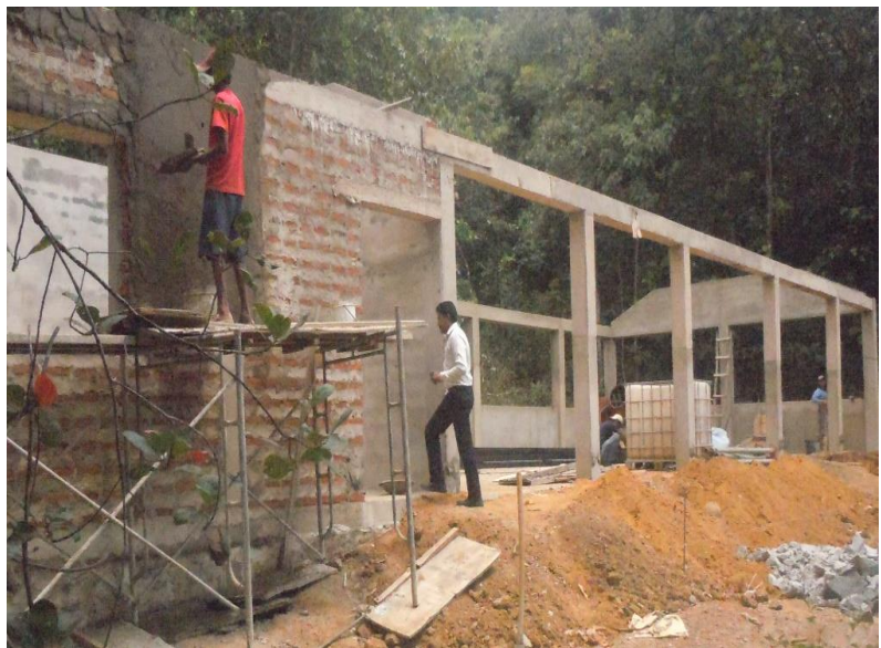
Construction of the in fieldoffice with a garage and a store room
