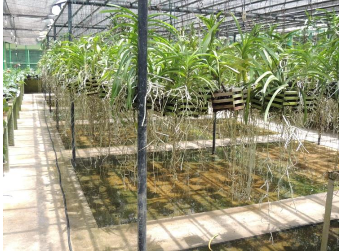
Arranging the earth to upgrade the Vanda Plant House of the Orchid Unit as to store the water
