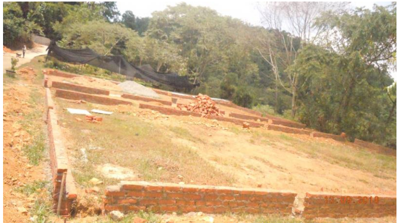
Construction of a shade house for plant nursery was initiated and activities were being carried out
