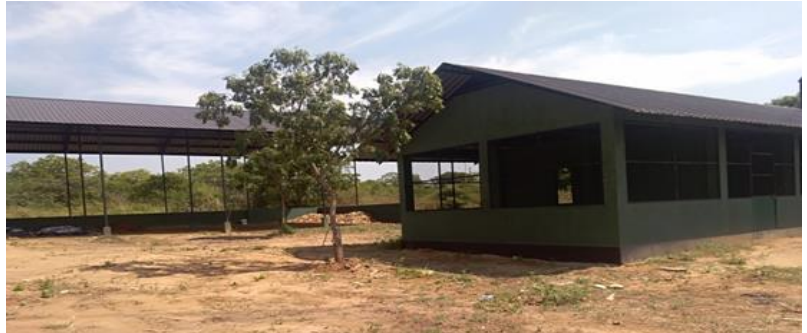
Newly constructed unit for waste water management in the garden
