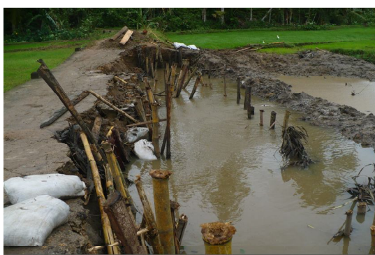
Washed away Road before the Reconstruction
