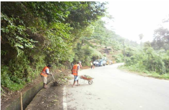
Lined Drain clearing near Km 47+700, LHS on Avissawella – Hatton – Nuwara Eliya Road
