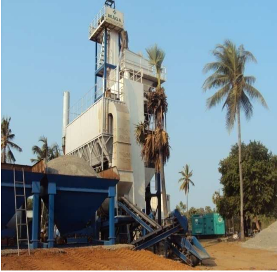
Asphalt Plant – Maga Engineering
