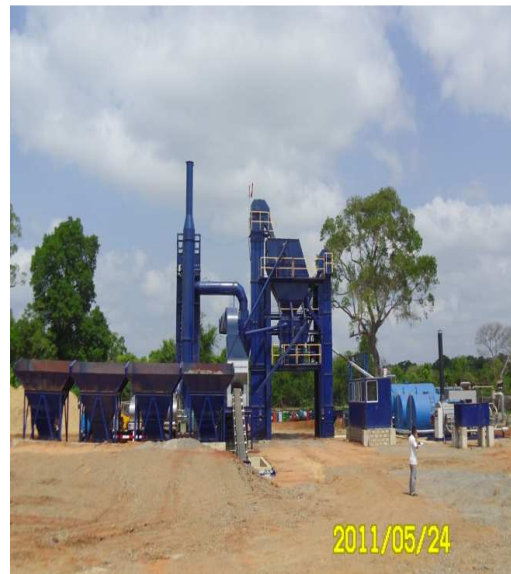
Asphalt Plant – A9 (CATIC-Eng)
