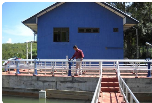
Part of the Godakawela WTP
