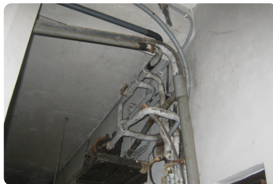
An example for unauthorized water consumption (By pass with pump installed)
