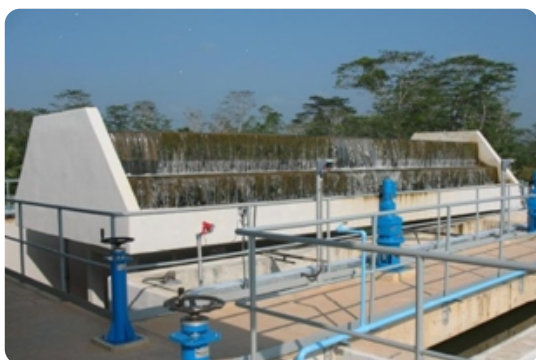
Baddegama Water Treatment Plant-
