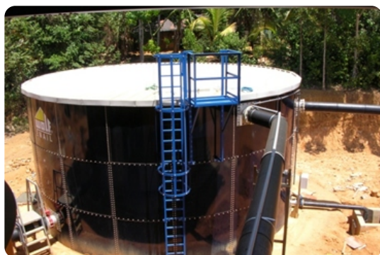
Water Sump in Weligama Water Treatment Plant
