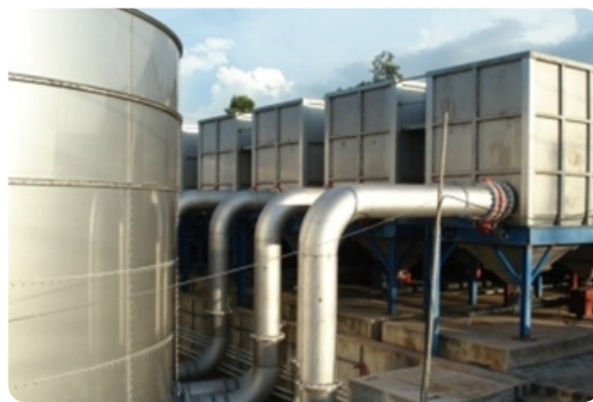
Negombo RO Water Treatment Plant
