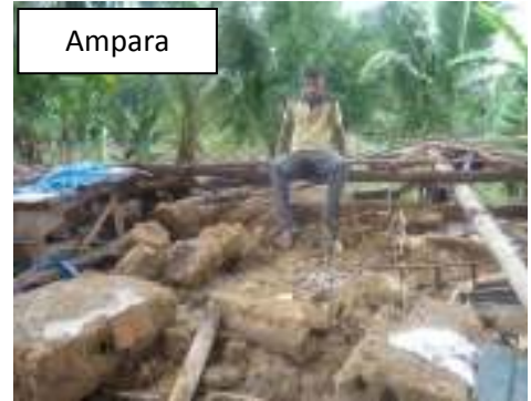
Completely destroyed house
