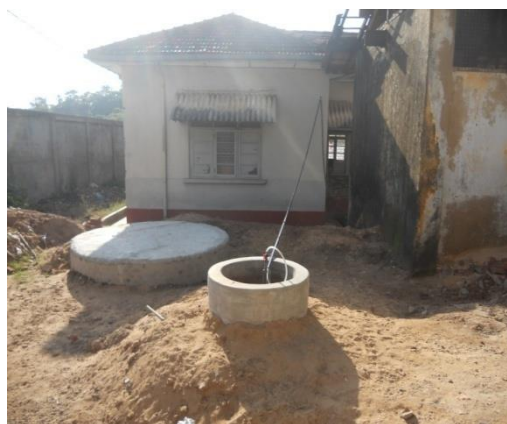
The biogas unit at the General Hospital,
