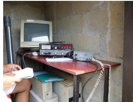
Fig No.23:Leakage Outlet Detectors and data recording system
