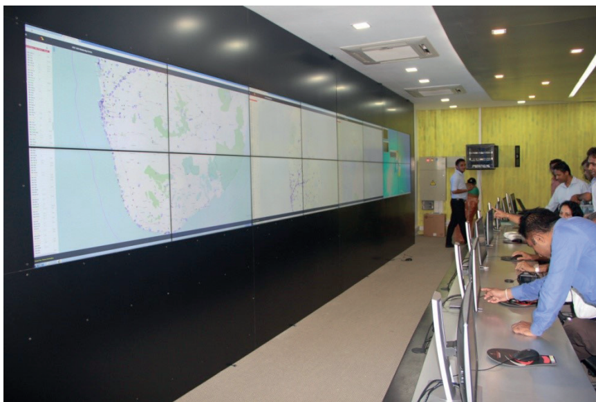
New GPS Control Room
