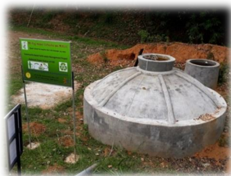
20m 3 Biogas Digester at Circuit Bungalow
