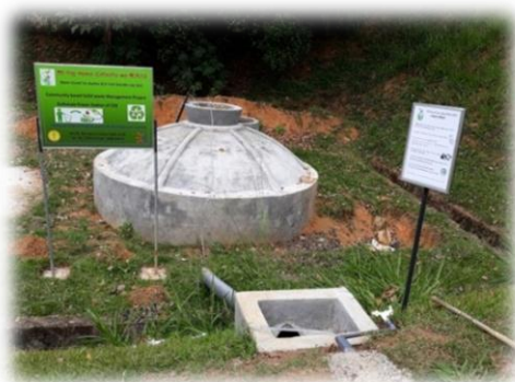
20m 3 Biogas Digester for Security Hostel
