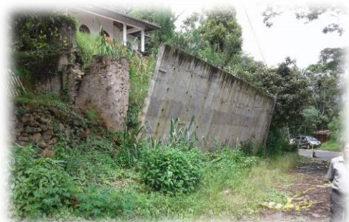
RC Retaining Wall Failure at Kothmale
