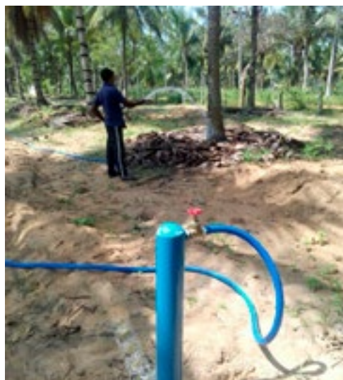
Newly developed hose irrigation system at the Pallama Genetic Resource Centre
