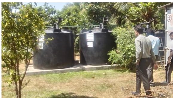
Welisara navy camp –Bio gas plant
