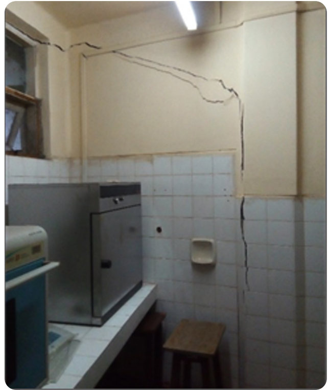
Cracked Walls at NIFS
