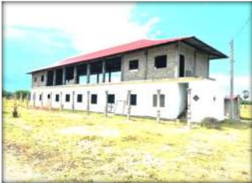
Completing remaining work of Dhamma school building at Welgam Raja Maha Viharaya in Trincomalee
