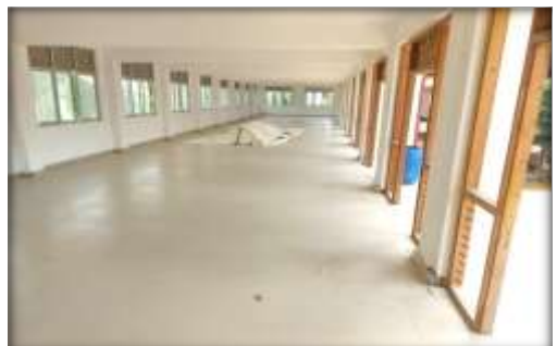
Completing work of Dhamma school building at Dedigama Kotawehera Raja Maha Viharaya in Kegalle district
