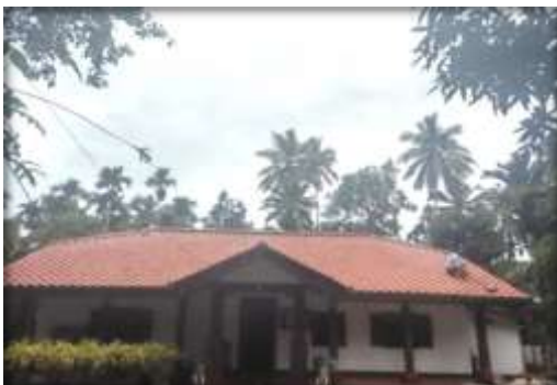
Renovating roof of the monastery of Meegammana Raja Maha Viharaya in Kandy district
