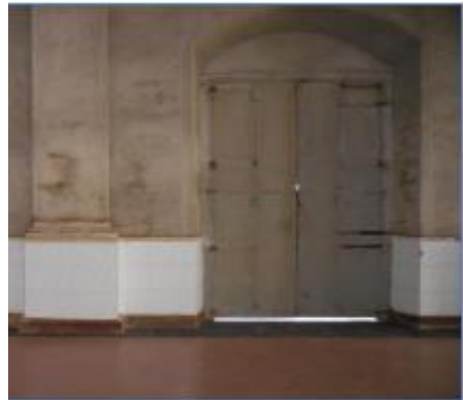
After the conservation of the plaster of the Duwa Sindrathi Church at Negombo, degraded due to salt
