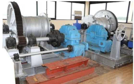
Gate hoisting system at Deduru Oya reservoir
