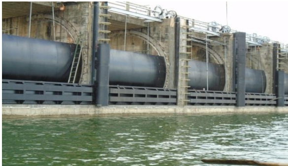
Water control gates at Rajangana reservoir
