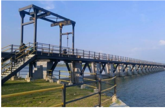
Water control gates at Thondamanaru barrage
