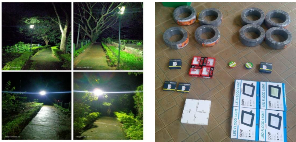
Entrusting repairs to the electrical lighting system of the Milapitiya Park for its protection
