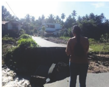
Breakage of Galmaduwa Road due to heavy rain – Kundasale Divisional Secretariat
