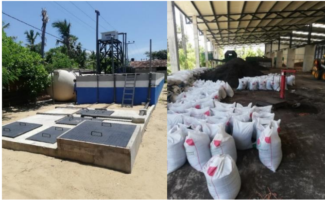
Kaththankudi Kawashima Yard and Sewerage system
