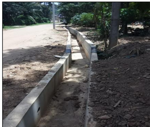
Construction of the sewerage system phase (ii) in the town. Katuwana. Weerakkuttigoda
