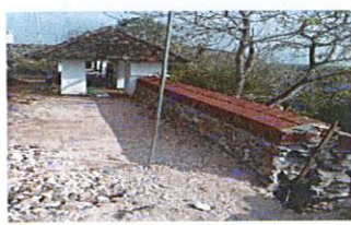
Conservation of the Stupa at Bihalpola Viharaya a portion of the rampart wall
