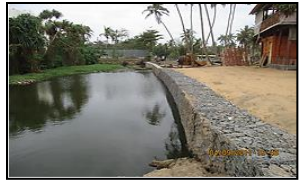
Proposed Construction of Gabion Structure under Storm Water Drainage System for Maha & Kuda Waskaduwa Area, Kalutara
