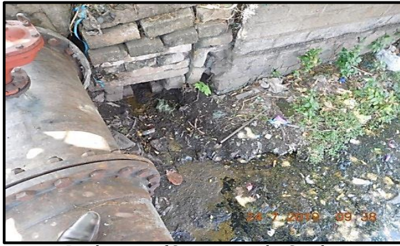
Discharging of Sewerage to the Canals
