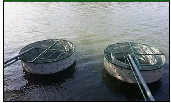
Pumping well for sprinkler system
