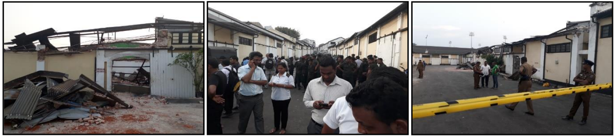
Collapse of building in Colombo on 14.02.2018
