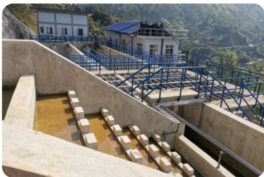
Ettampitiya Water Treatment Plant
