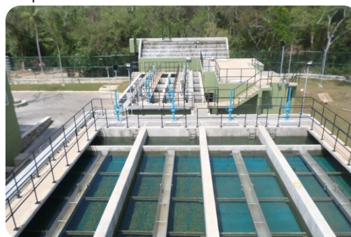
Water Treatment Plant - Chilaw
