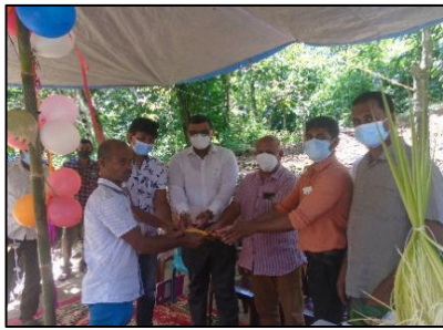
Laying the foundation stone for the construction of a house under the 'Home for Poor You' program in Handungala Estate, Pasbage Korale Divisional Secretariat under the patronage of the Hon. Chairman of Nawalapitiya Urban Council and the Hon. Chairman of Pasbage Korale Pradeshiya Sabha.
