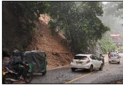
Earth slip at pahala kadugannawa of the Kandy-Colombo road due to bad weather condition prevailed in November, 2021.
