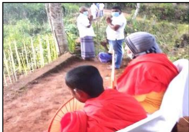
Laying foundation stone to rehabilitate the Dunuwila Lake under the patronage of Hon. Governor of the Central Province and members of the Akurana Pradeshiya Sabha including the Chairman.
