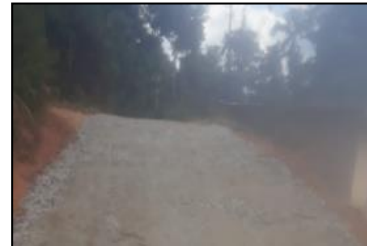
Development of the entrance road near the Wembliwatta Community Hall in the Uduwara Divisional Secretariat Division under the Special Needs Village Development Program implemented by the Central Provincial Council.
