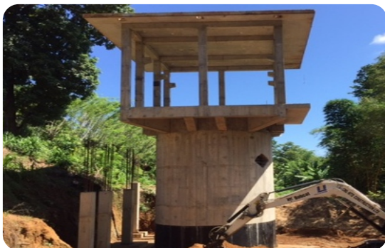
Intake Well and Pump House
