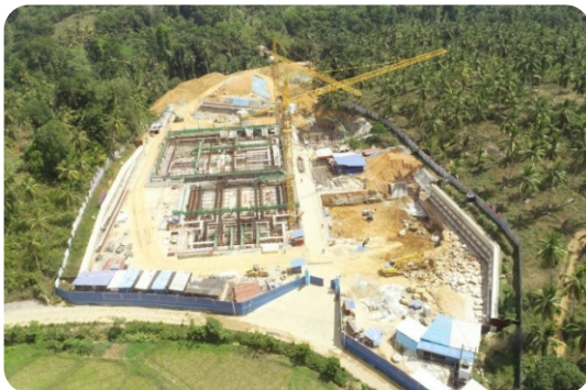
Water Treatment Plant at Karasagala
