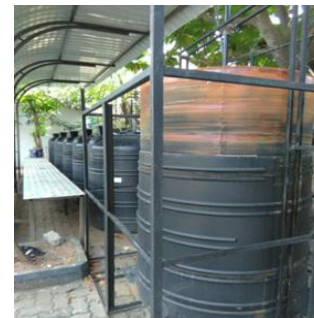
Biogas Digesters at SLIDA
