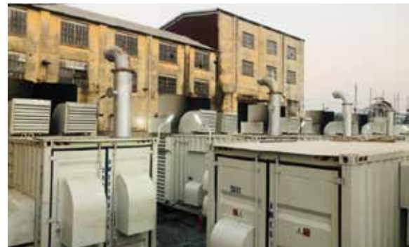
1MW generators at Kolonnawa site -02
