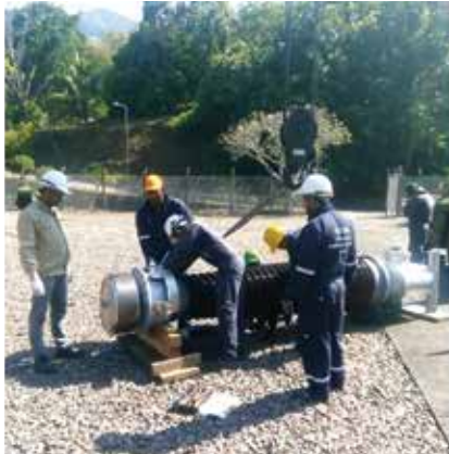
New CT before installation
