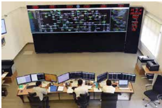
Figure Tr-3: System Control Centre
