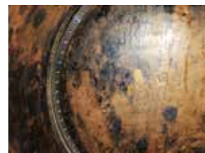
MIV Blade at close position before repair
