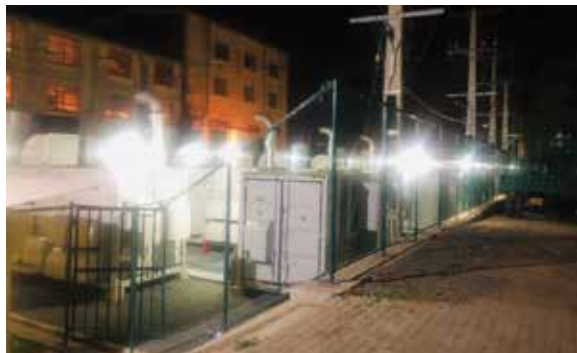
1MW generators at Kolonnawa site -02
