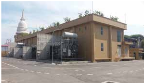
Colombo L Grid Substation
