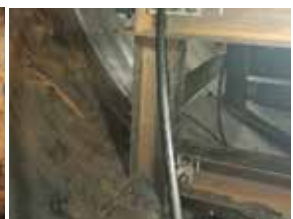
MIV Blade Seal before repair
