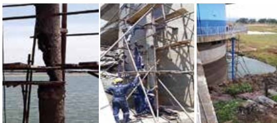
Corroded steel pipe
