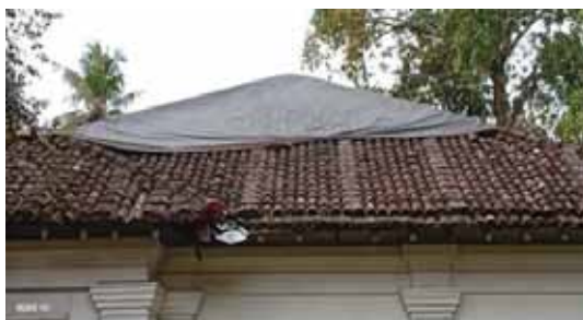
The condition of the roof of the office section of the Mahawalawwa Hall before renovation
