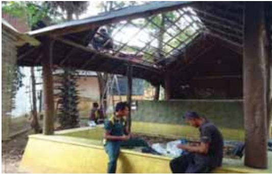
The condition of the stall roofs before they were repaired
