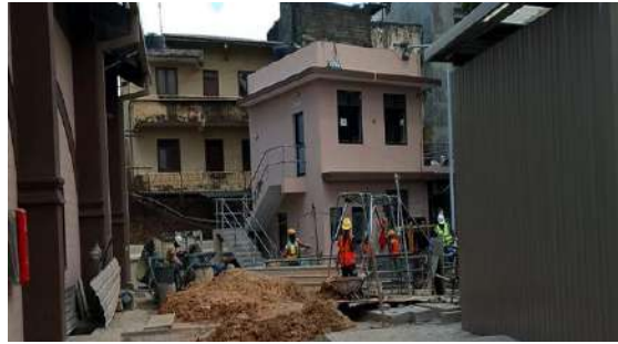
Maligawaththa Pump station
