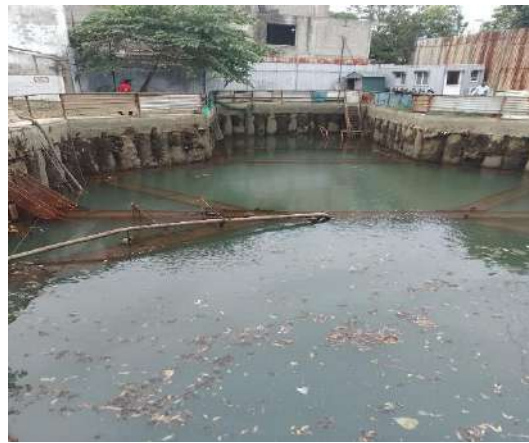
Thalakotuwa Garden Pumping Station
