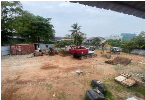
Kirula Pumping Station
