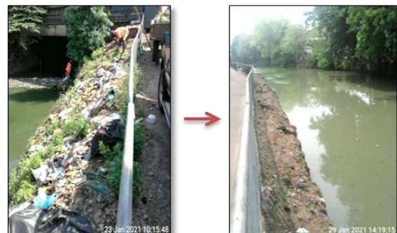
Disposal of Solid waste into Canal Bank
