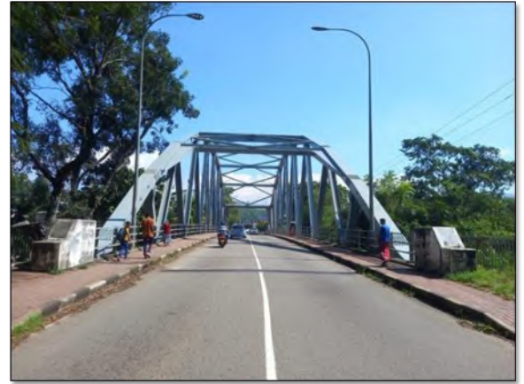
Figure 2-7: Repainting of 1/1 on Rathnapura – Palawela – Karawita road (Muwagama bridge) (Consulting with specifications)
