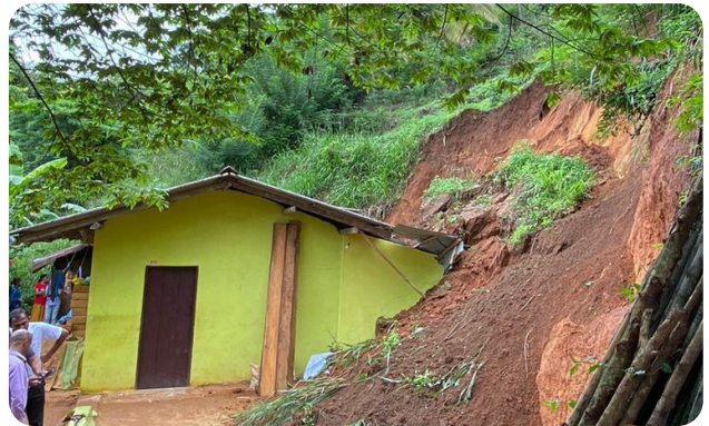
Cutting Failure at Wathuliyadda - Kandy
