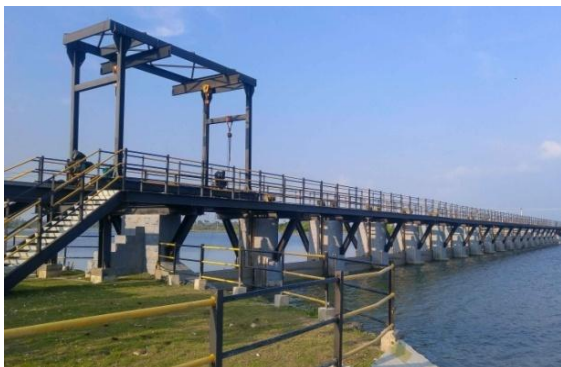
Water control gates at Thondamanaru barrage
