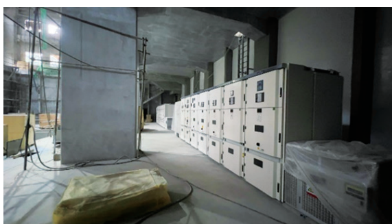
Electrical and Electronic installation in Power House
