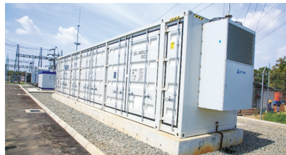
Battery Energy Storage System – Hambantota
