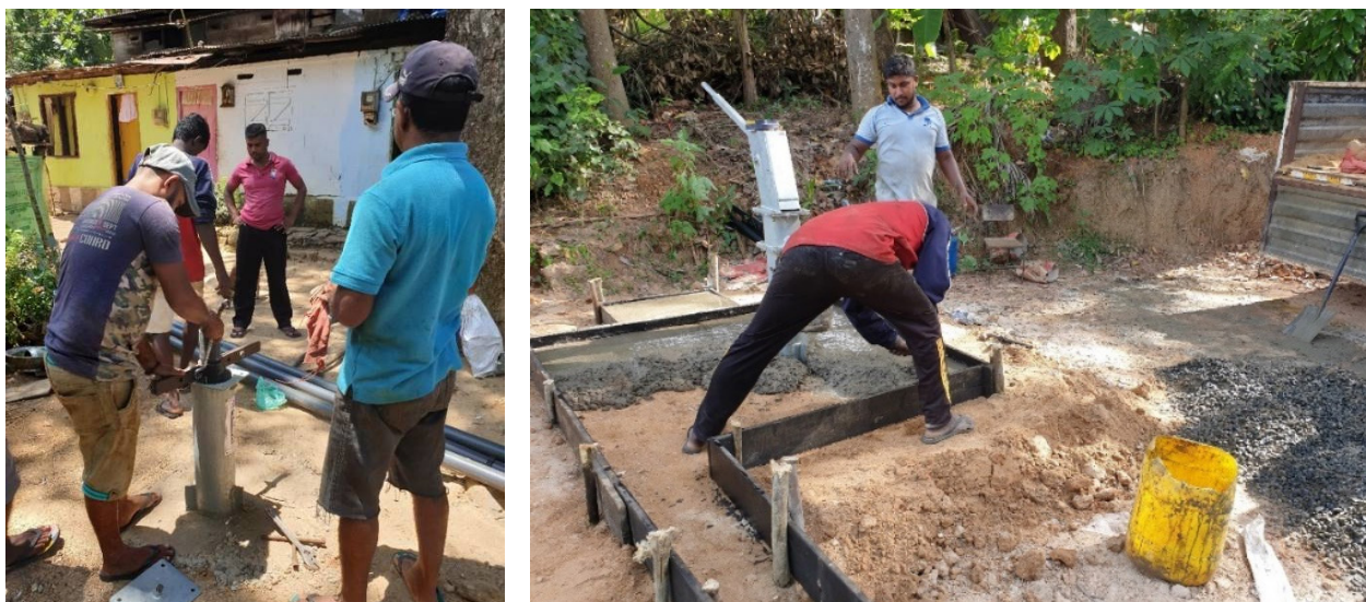
Figure 32: Hand pumps installed in Matara and Bemmulla areas
